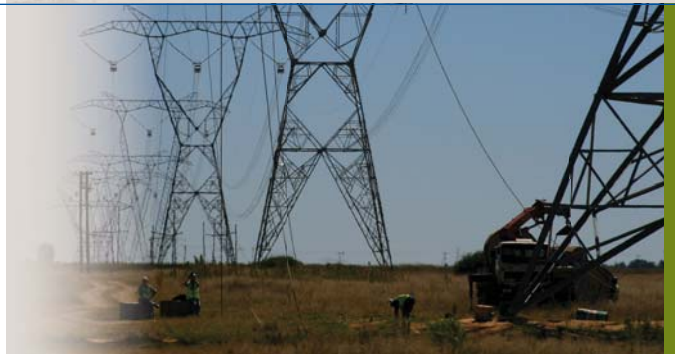
High-voltage power lines are strung in the Free State.
